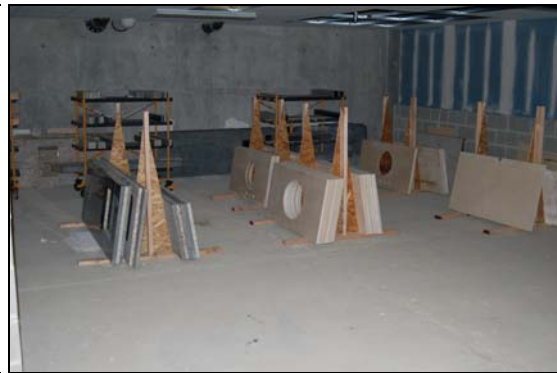
On-site Stored Materials – fabricated stone kitchen and bath countertops, well organized, stored under cover well protected from weather and vandal exposure
