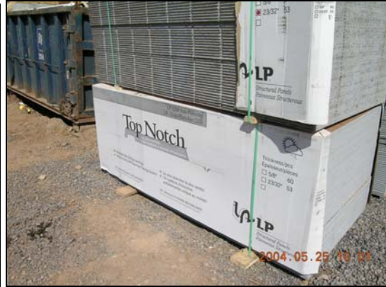
On-site Stored Materials banded and partially protected sheets of OSB-subflooring for multi-family housing project, bottom of pile is only supported off crushed stone using 2x4 wood studs – any localized standing water will be ‘wicked’ into sub-flooring sheets
