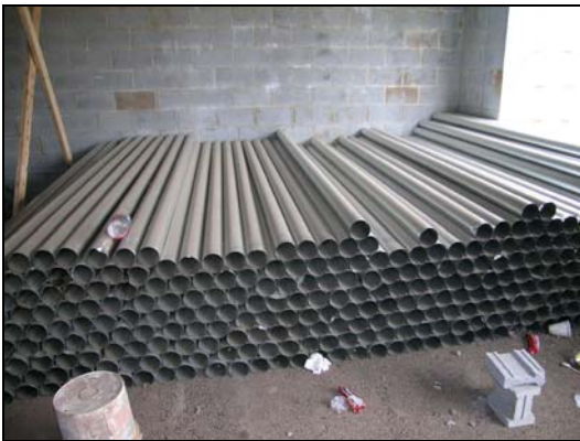
On-site Stored Materials – fabricated metal bath and kitchen exhaust ductwork – generic ductwork is piled on earth under cover in future parking garage located under new multi-family housing structure.
