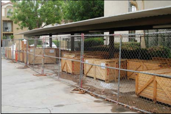
On-site Stored Materials under carport behind temporary fencing; crates of fabricated kitchen & bath vanity stone countertops, material will not be installed within next (30) days but order is reported by Contractor to be complete & adequate.
